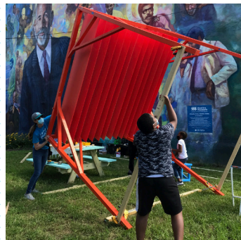
Flip structure onto its side (here's why we need the leg bracing.)
