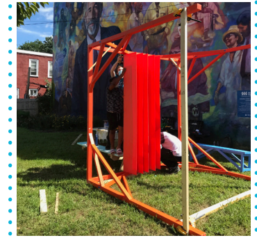
Use clamps or screws to attach temporary bracing to support the legs.
