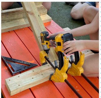
Tip! Use a clamp to keep the diagonal from moving left or right.
