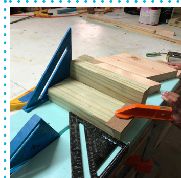
Align these "L" blocks 11" (or two 2x6 cut-offs) from ends of the seat slats.
