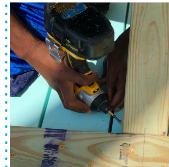
Pre-drill and toenail a screw on each side of diagonals at table top.
