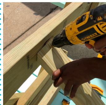
Mark and center diagonals to legs and top. Use 18g nailer to pin in place.
